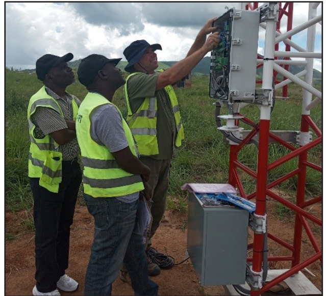
Meteorological Engineers during installation and onsite training at Bakili Muluzi International Airport
