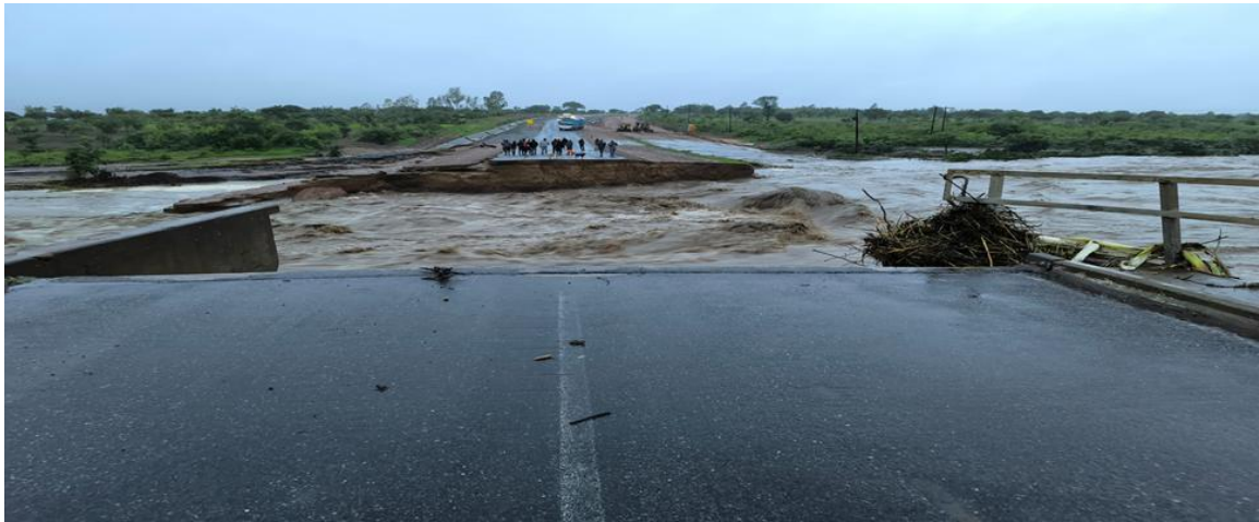
Figure 43: Floods swept away Mpasadzi Bridge: National Online (31 December 2025)
