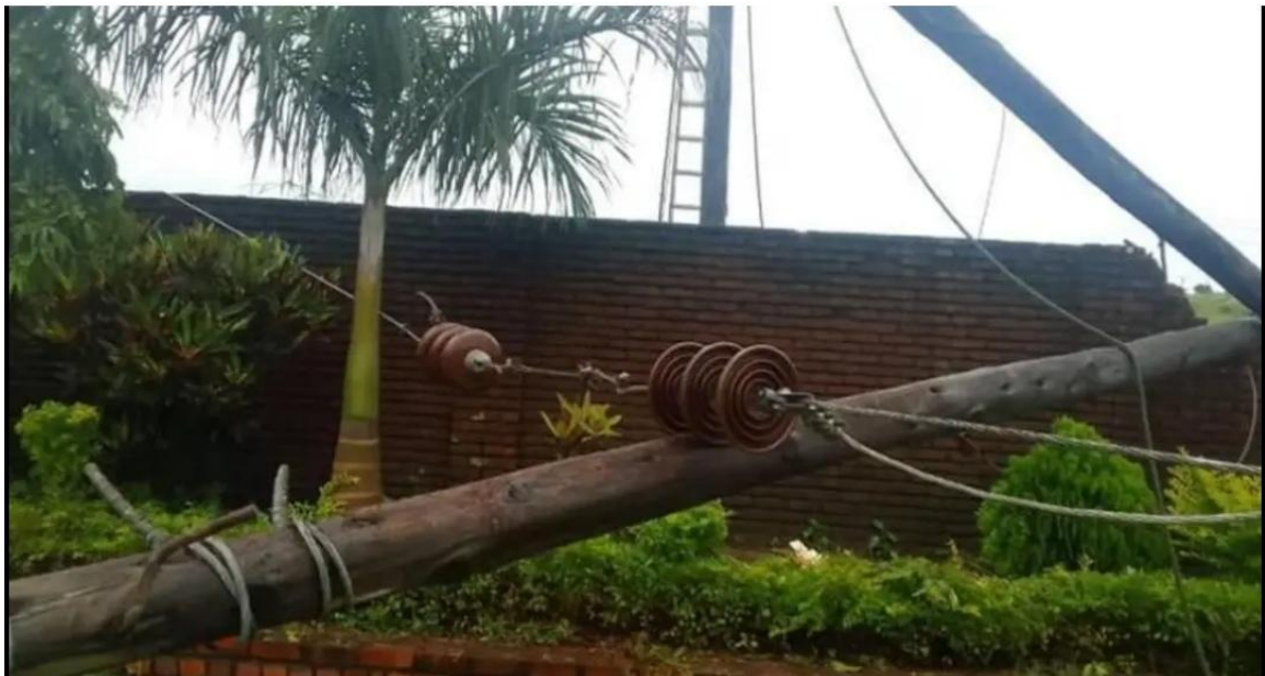
Figure 44: Electricity pole that fell due to heavy rains and strong winds in Lilongwe on 10 December 2025. Zodiak Online. (2025, 12 10. https://www.zodiakmalawi.com/ )
