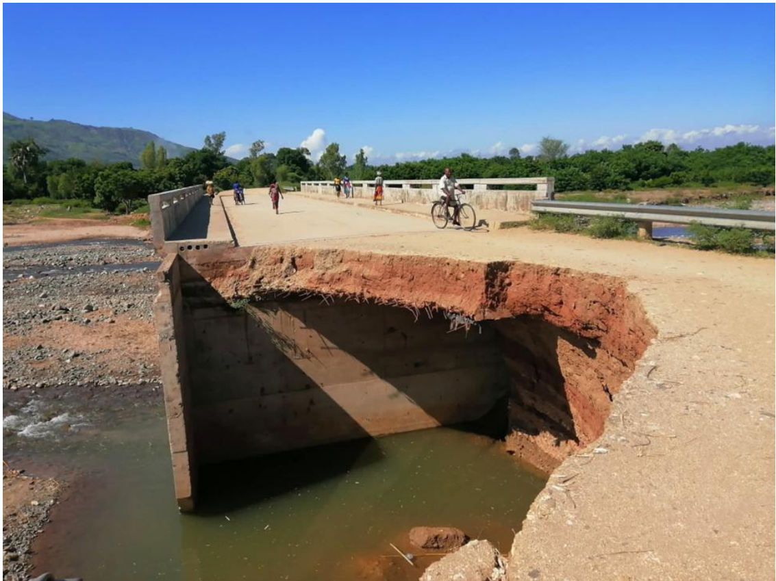
Figure 45: Chizimbi bridge Thabwa-Fatima road partly damaged disrupted ferrying of patients to Queen Elizabeth Central Hospital in Blantyre for tertiary care (Zodiak Online 26 March 2025)
