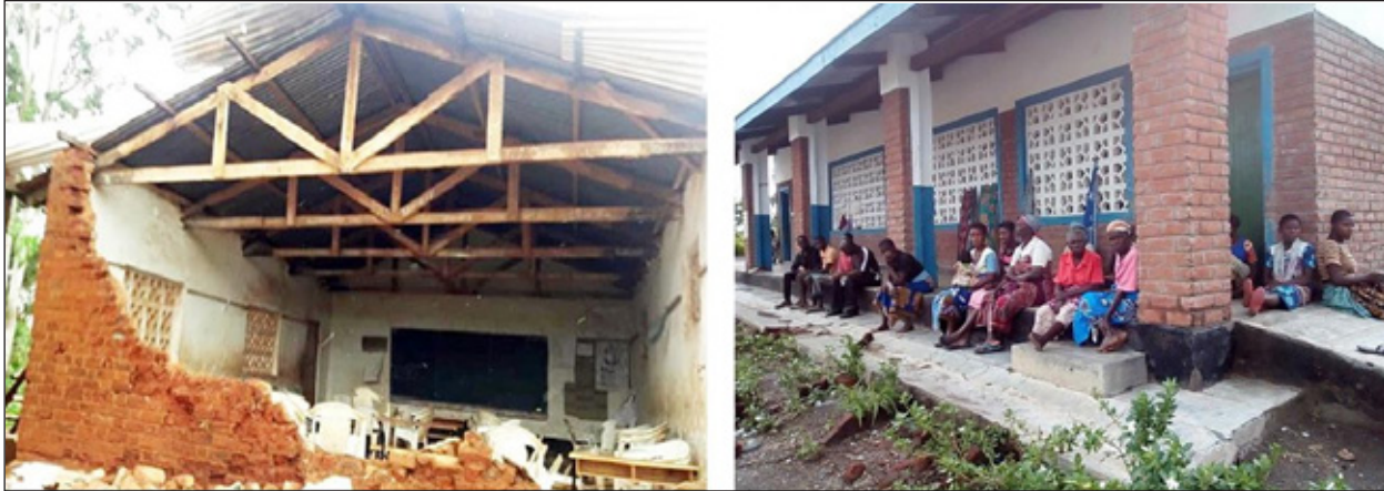
Figure 28: Left: Classroom damaged. Right: Families shelter at a local school in Neno District during by cyclone Ana (Partners In Health, 2022).
