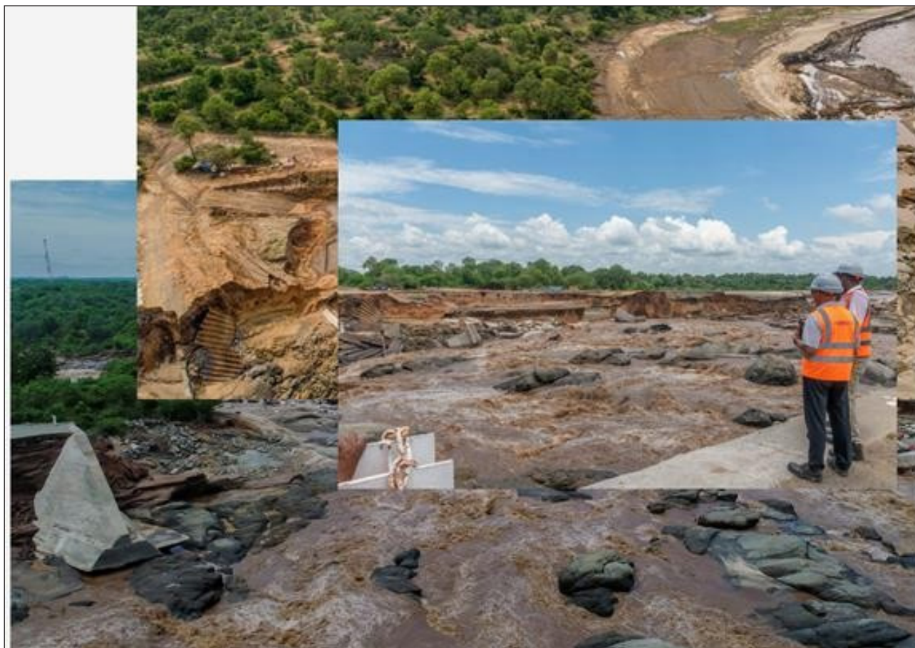
Figure 24: Kapichira power station dike, extensively damaged by Tropical storm Ana in January 2022 (EGENCO, 2022)
