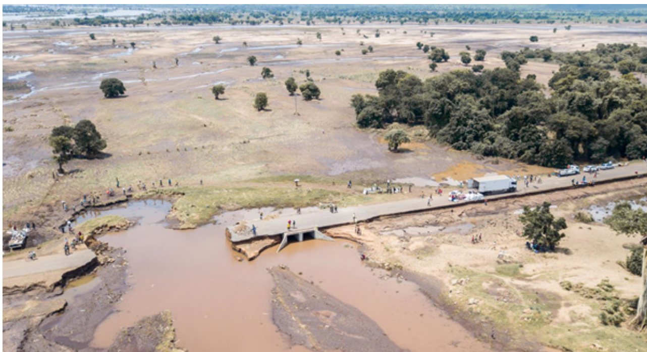
Figure 21: The M1 road in Chikwawa district was damaged by the floods
