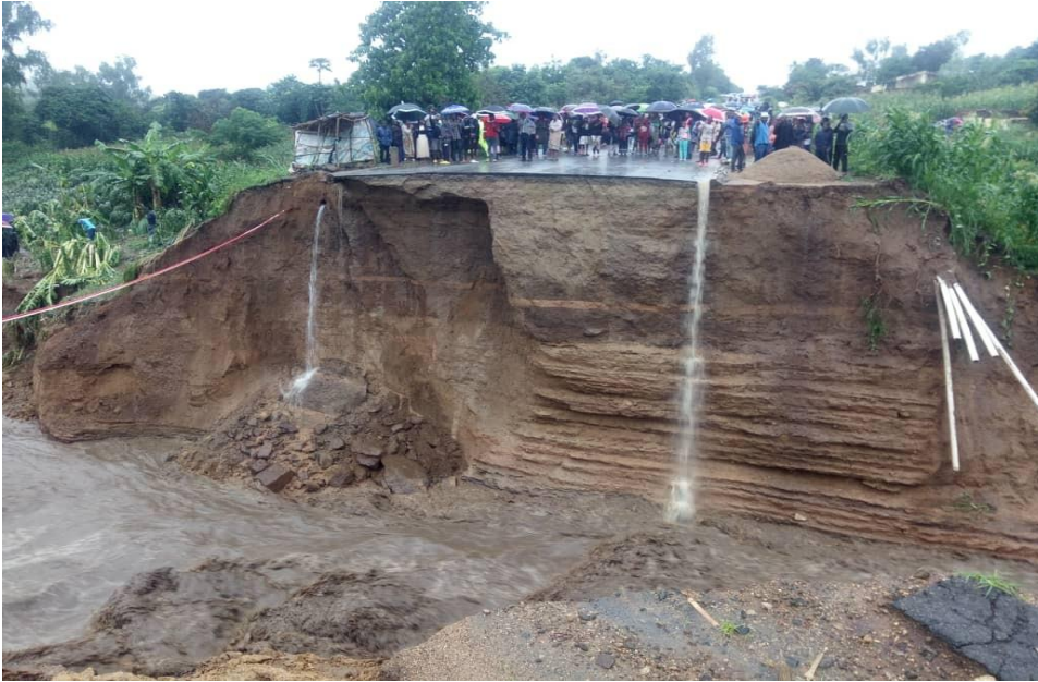
Figure 31: Road washed away by heavy rains in Machinjiri, Blantyre
