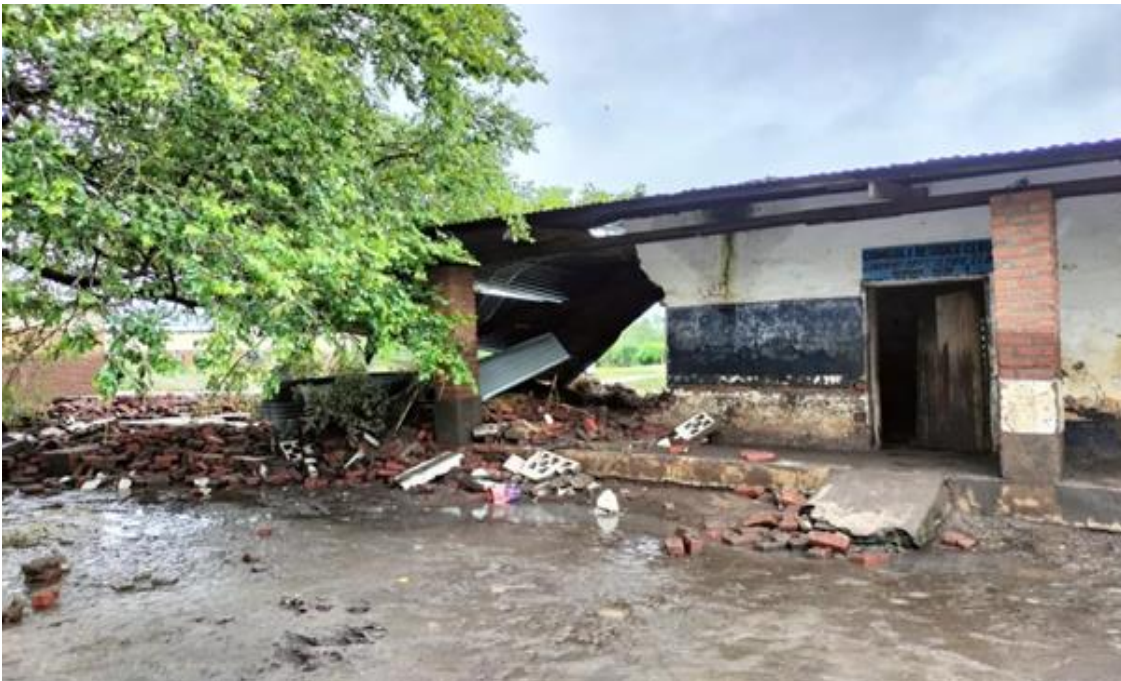
Figure 35: Chingoli Primary School In Mulanje was affected by tropical cyclone Freddy on 12th March 2023 (Siula, 2023)
