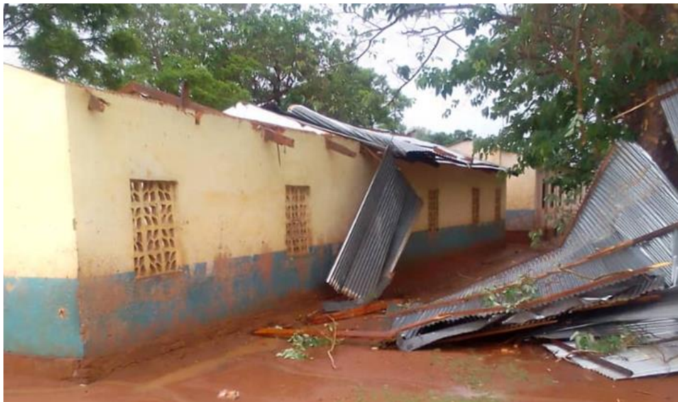
Figure 29 Roof blown off by strong winds at Bwengu Primary School in Mzimba District in December 2023.
